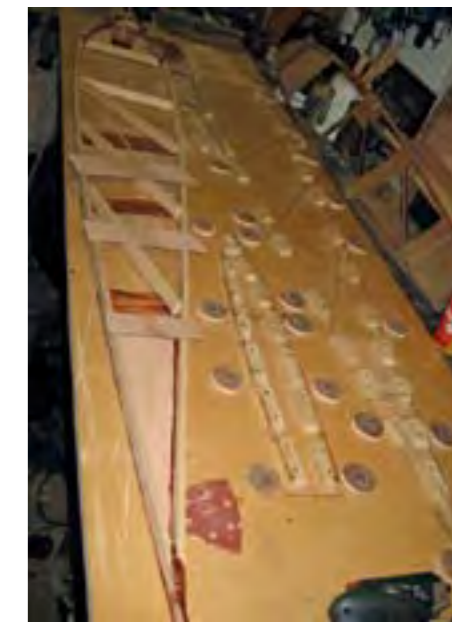
Rib jig can be set up indoors to allow the Aerodux to cure
