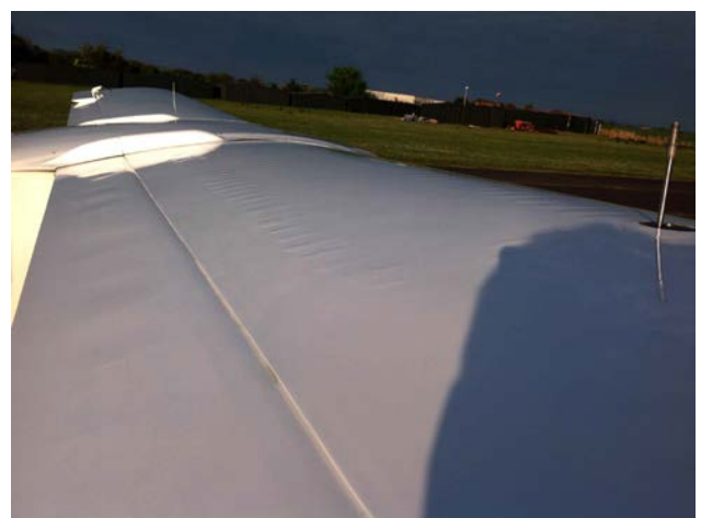
Fig 2. Though difficult to see in this picture rippling can be seen in the top surface of this J400 wing. The recent AIL withdraws any previous approval for Mogas use.
